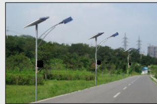
Solar Street Light
